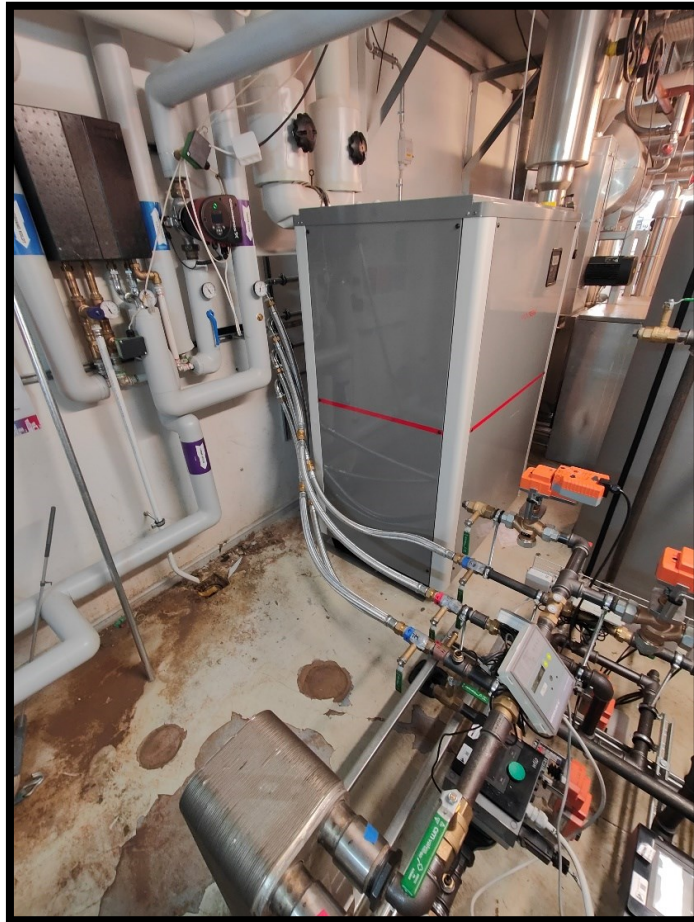
Figure 10 – Heat pump installed with pumping station.
