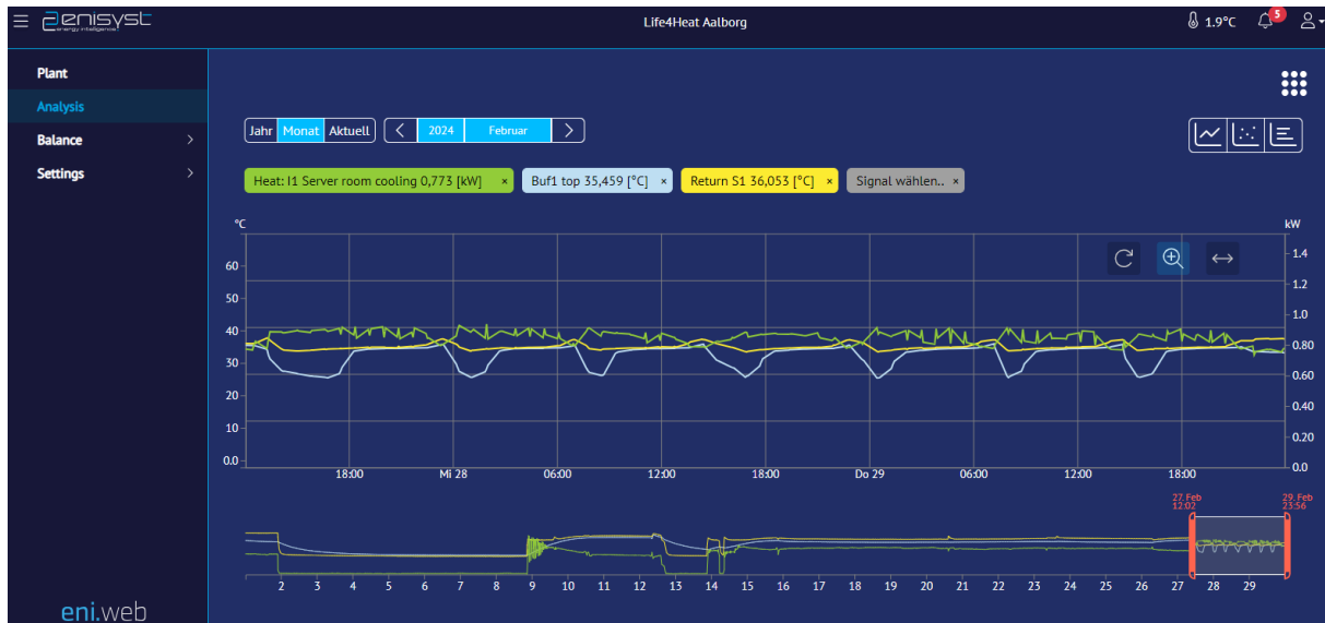
Figure 12. The SCADA interface developed by ENISYST.
