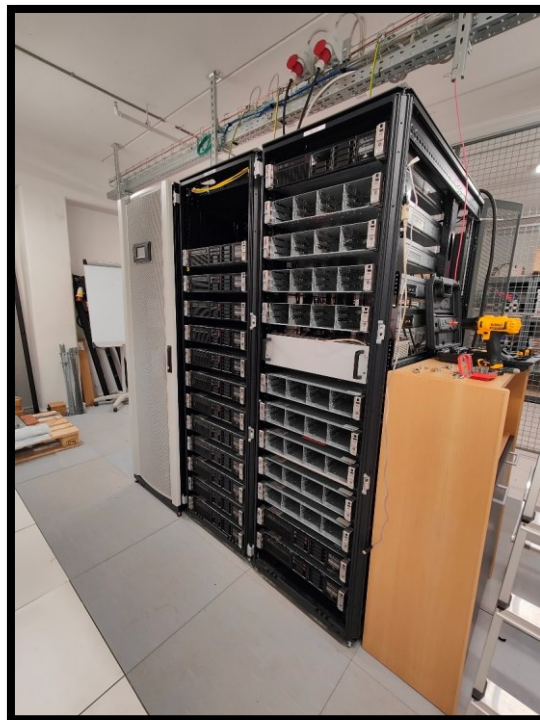
Figure 5 – Configuration of server racks in demo room.
